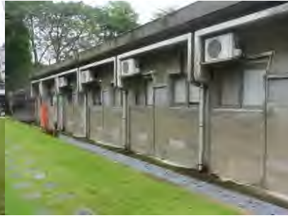
8.東向立面左半邊室外機外掛
